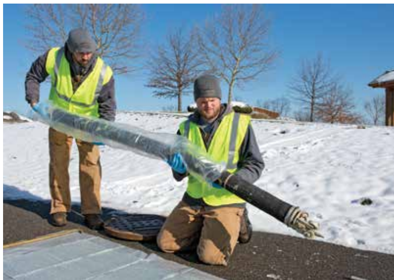
Maintenance workers Jeremy Gruelle (left) and Bryce Meier prepare a pipe patch for a sewer line repair.
