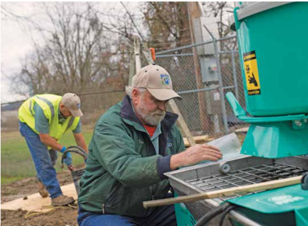
Top: Putnam Public Service District maintenance crew member Jeremiah Campbell applies grout to a manhole wall at Scary Creek Industrial Park in Scott Depot, West Virginia. Above: Tom Forth pumps grout through the Step Up 120 (Imer Group) grout pump and spray machine while his crew sprays the inside of a manhole.
