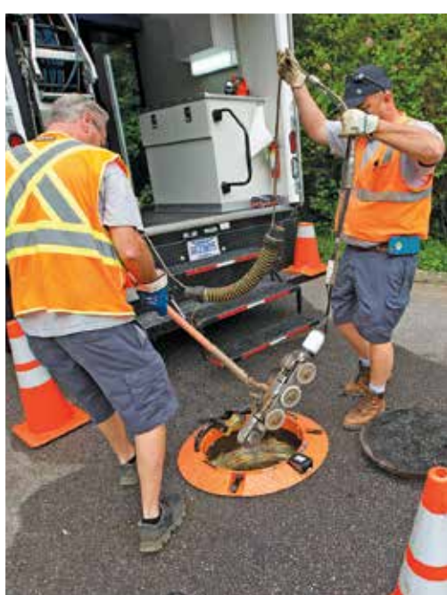
Mike Jones (left) and Gary Cantrell lower a CUES camera into a manhole for a sewer line inspection.
