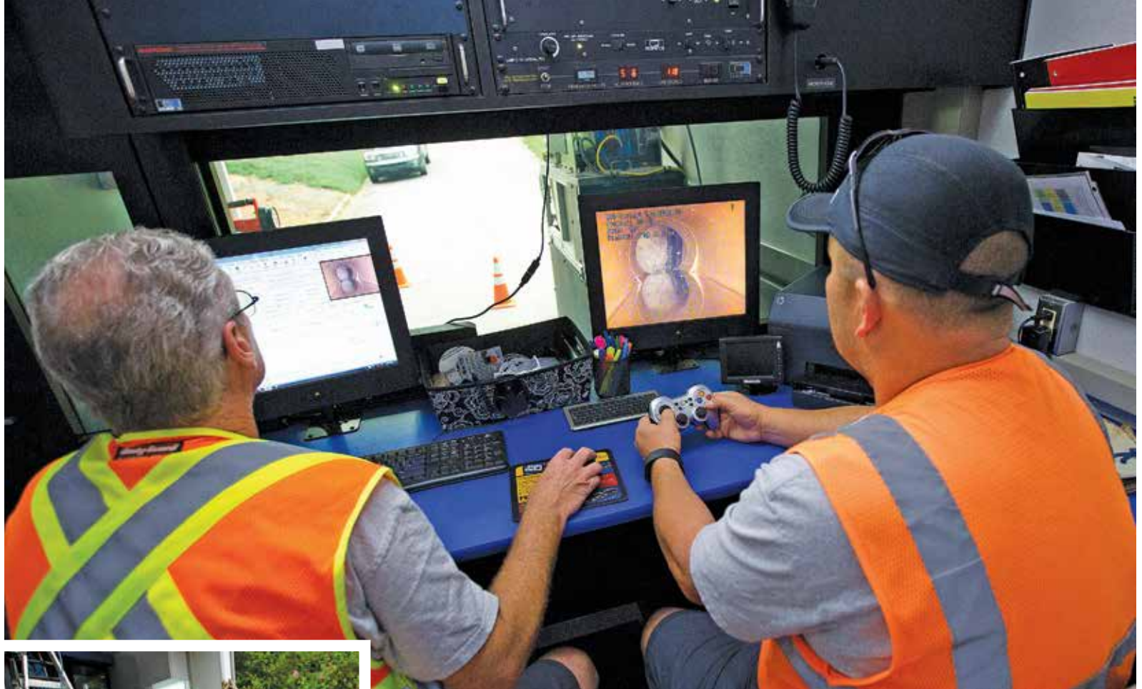
Technician Mike Jones (left) and TV crew leader Gary Cantrell run a sewer line inspection from the control room of the CCTV van.
