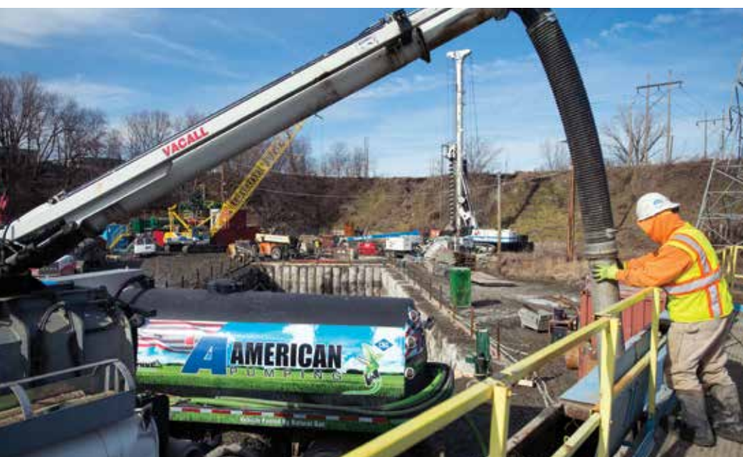
Backlund Plumbing technician Jamey Severn guides the boom from a Vacall AllExcavate hydroexcavator into a Rain for Rent dewatering tank at the Leavenworth Lift Station replacement project in Omaha, Nebraska.
