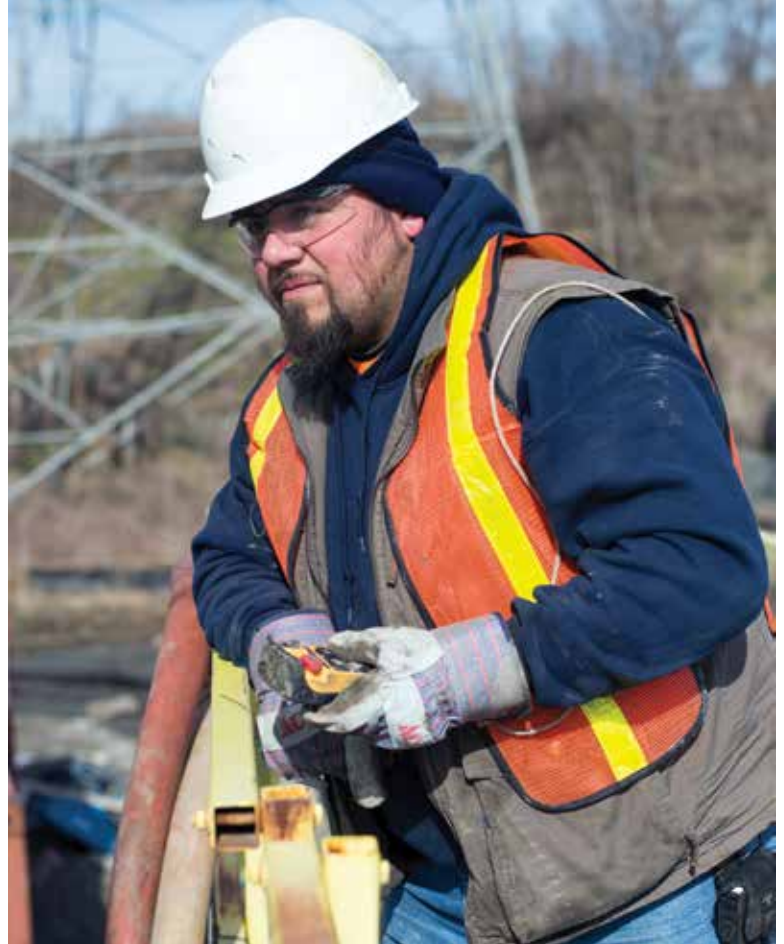
Backlund Plumbing technician Johnny Compos uses a remote control to guide a hydroexcavation boom at the Leavenworth Lift Station.
