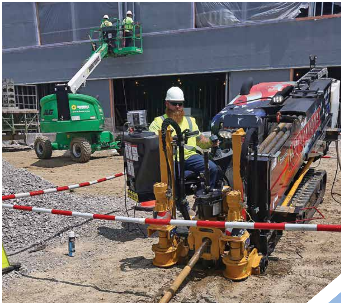
CST Utilities operator Nick Gilbert uses a Vermeer 20x22 directional drill while boring for new electrical lines for a new apartment building.
