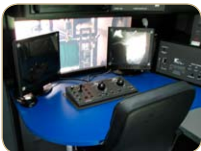
VIEWING ROOM FLAT SCREEN MONITORS & INDIRECT LIGHTING
