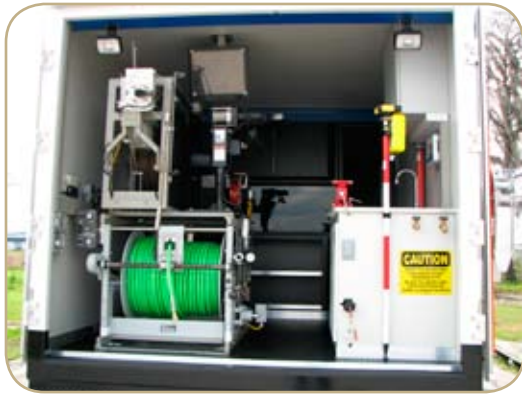
EQUIPMENT ROOM WITH LARGE VIEWING ROOM WINDOW
