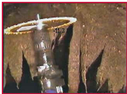
Small, thin roots were easily cut with the 6.5-inch saw blade mounted on an air drill. These roots were not suspected to be the cause of pipe surcharging.
