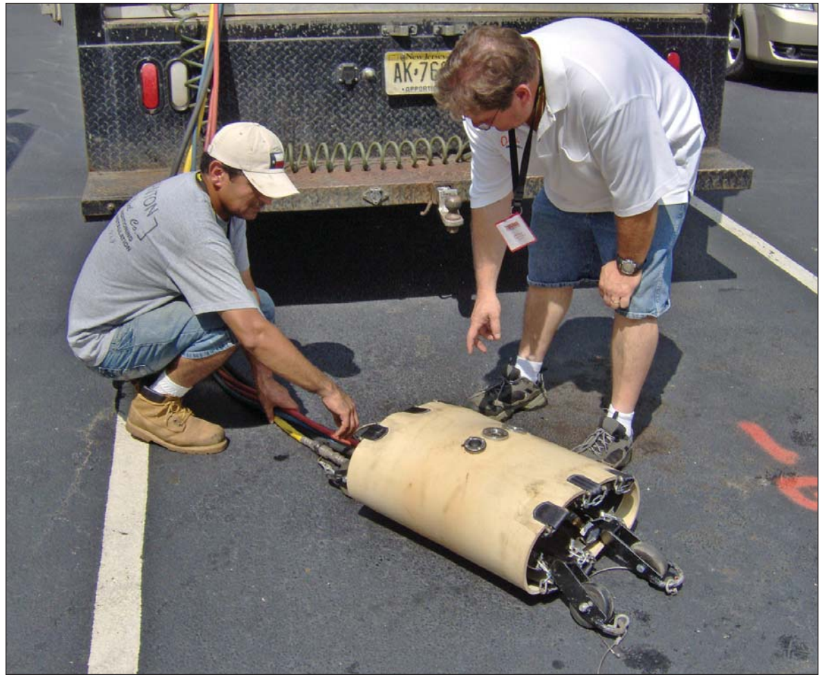
Antonio Rocha (left) from Oswald Enterprises Inc. in Belford, N.J., attaches hoses that deliver air and grout to the 14- by 23-inch elliptical packer custom-built by Logiball Inc. Project manager John Read oversees the process. (Photo courtesy of Oswald Enterprises Inc.)
